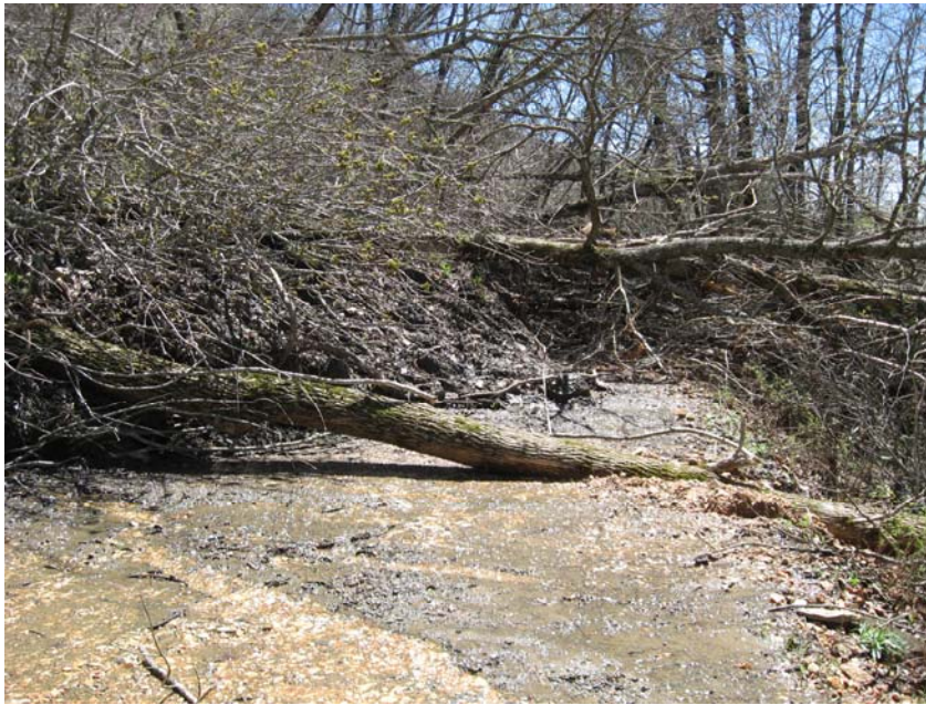
View (north side) of landslide covering road. Notice water flowing from slide onto road.
