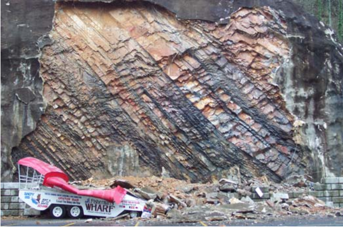
Gunnite collapse in 2005 that destroyed duck.
